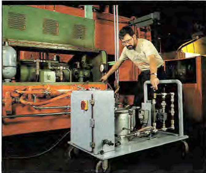
Technician connects advanced portable oil filter to plant machine. The filtering equipment has the capacity to return oil to better than new condition with regard to particulates.
