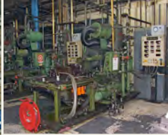
Screw Compressor Test Stand
